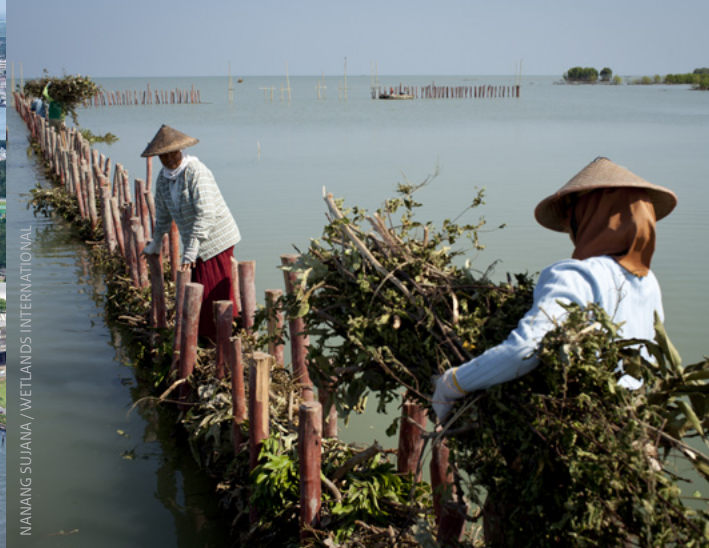
Indonesian people building dams of natural materials to help mangroves get re-established
